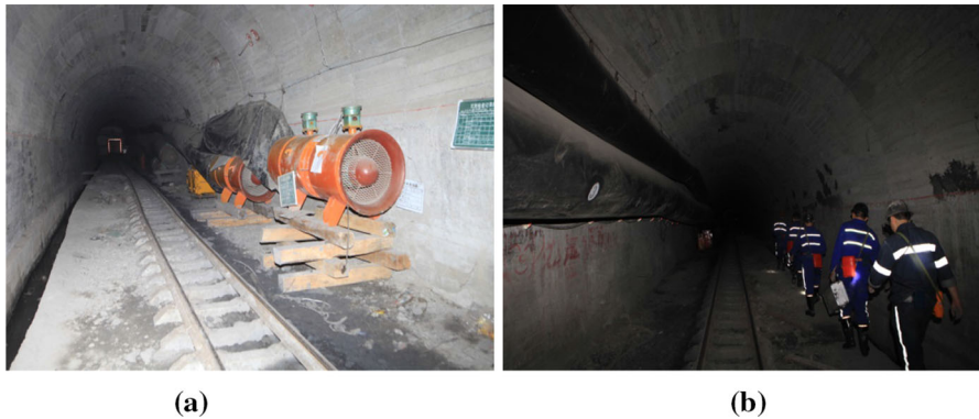
Fig. 18 Support effects in the field. a Section 1 and b section 2
