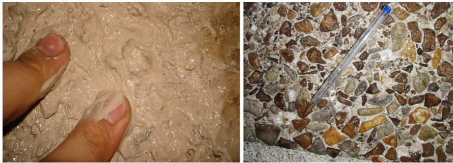
Fig. 7 Examples of concrete deterioration at the Zagros tunnel which resulted in the softening of concrete matrix, swelling and spalling
