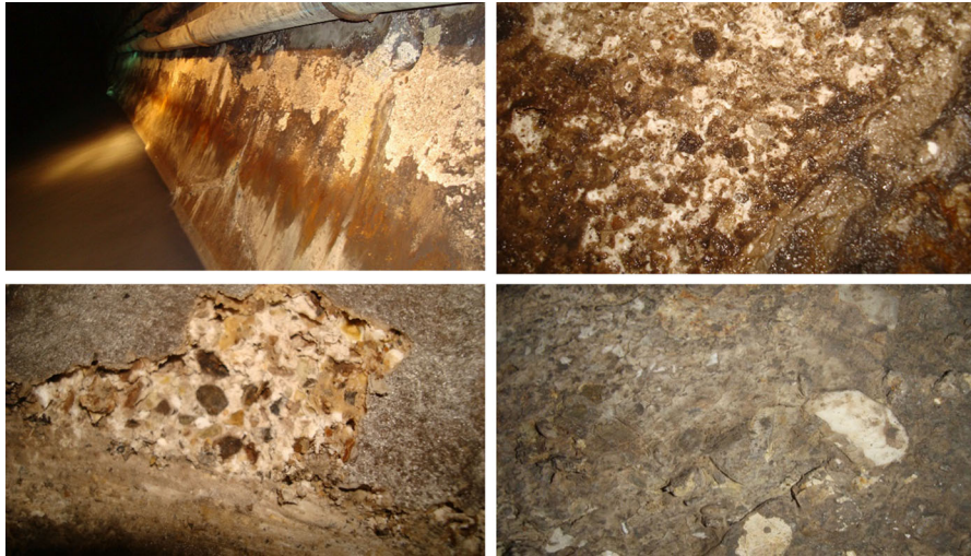
Fig. 6 Typical examples of the segmental lining deterioration (spalling and swelling) at the Zagros tunnel
