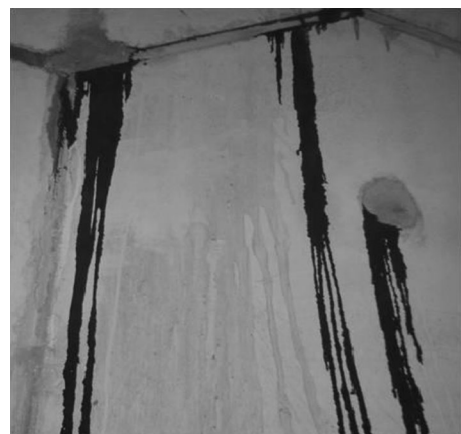
Fig. 8 Seepage of organic bitumen into the Zagros tunnel from segments' joints. (Courtesy of Mirmehrabi et al. 2010)
