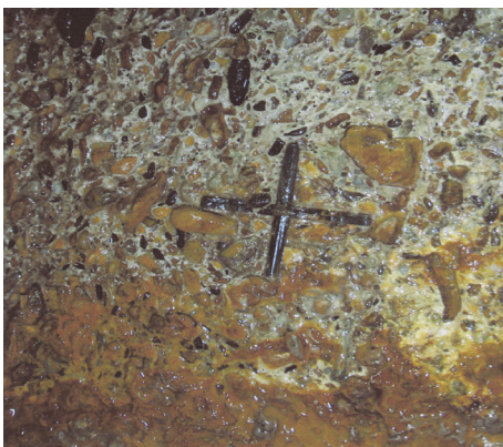
Fig. 16 Deterioration of the concrete cover and the exposed reinforcement, at the Zagros tunnel
