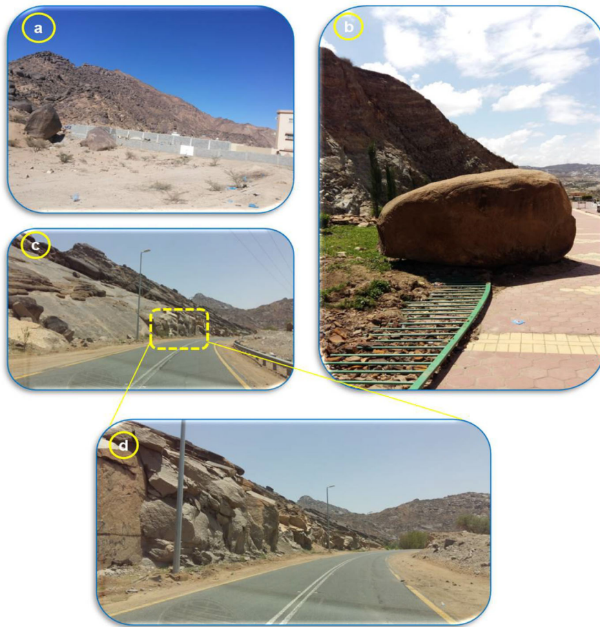
Fig. 9 a, Field photograph showing the rock falls in central part of Najran, b, in highway between Najran-Abah road; and c, d slope failure in Najran Habona road
