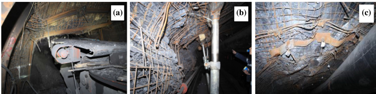
Fig. 4 Combined support scheme with bolting-cable-beam-belt support failure. a Roof subsidence, b sidewall bulging, c severe roof support deformation
