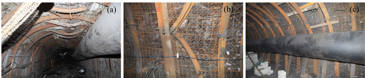
Fig. 2 Support failure with I-steel shed and metal mesh. a Arch bending, b disjointing at the welded points on the sidewall, c foot moving inward, overall integrity reduced
