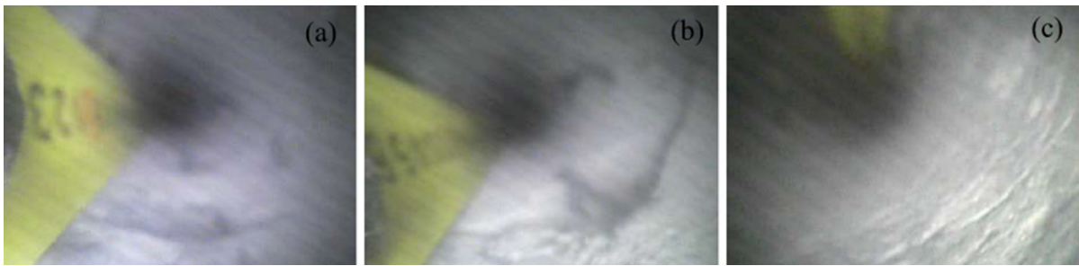
Fig. 7 Peephole observation of fissures in tunnel roof rock mass. a 1.5 m away from the peephole, partially fractured, b 2.8 m away from the peephole, partially fractured, c 3.5 m away from the peephole, good rock integrity
