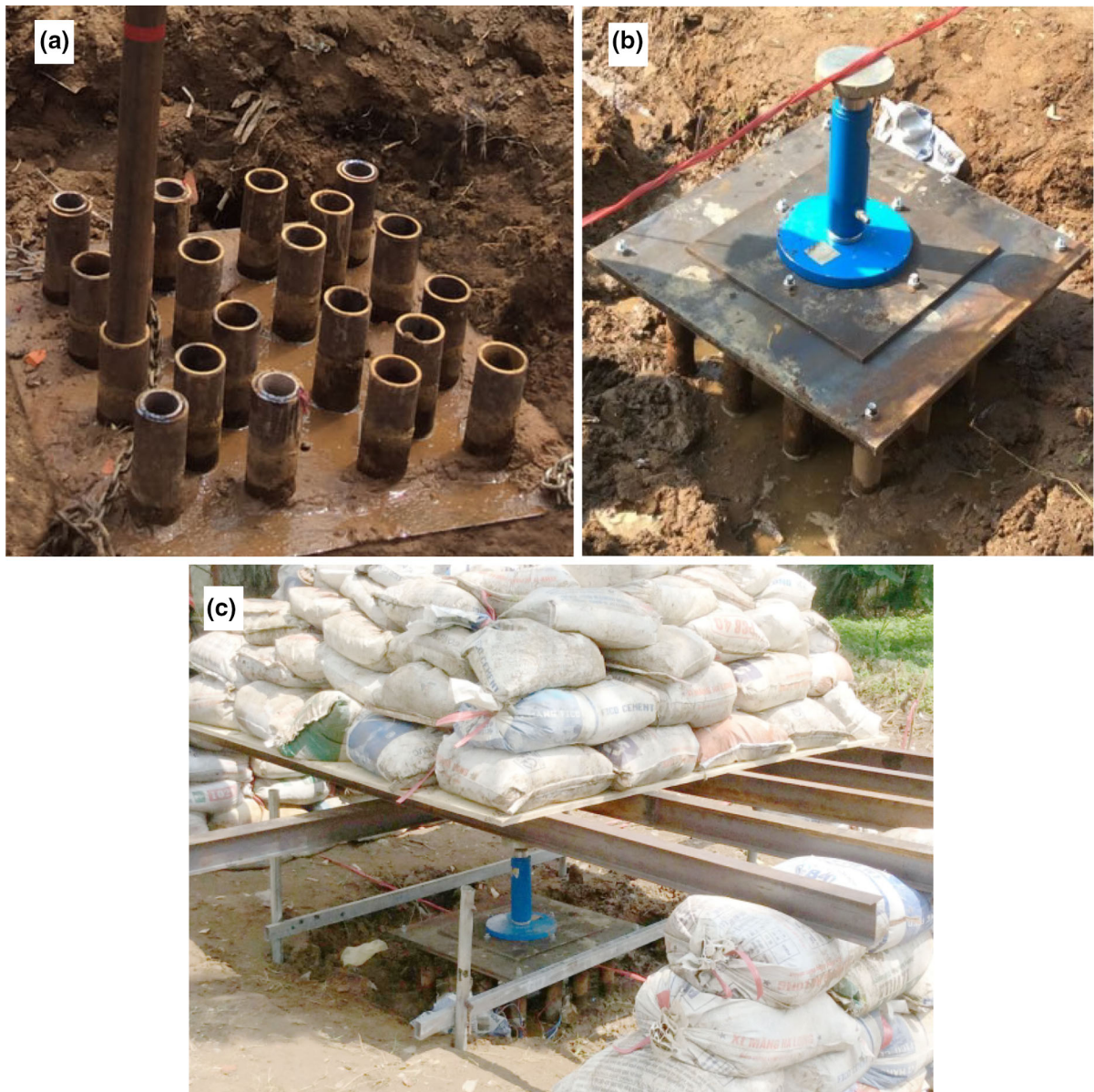
Fig. 4 Installation and test of the pile groups: a installation of 16-pile group, b Construction of rigid cap and c Set-up of kentledge system (Authors' photo)
