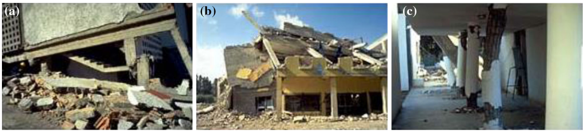
Fig. 2 Recorded building damages during 1980 El Asnam earthquake. a Medical clinic. b Algerian gallery store. c Primary school canopy
