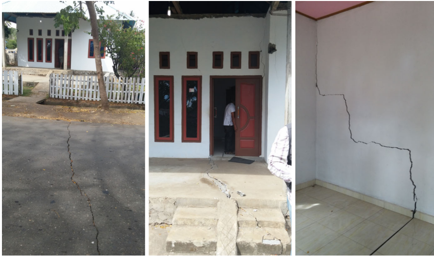
Fig. 8 Crack on the road that continued towards adjacent residential buildings resulting in damage to floors and walls
