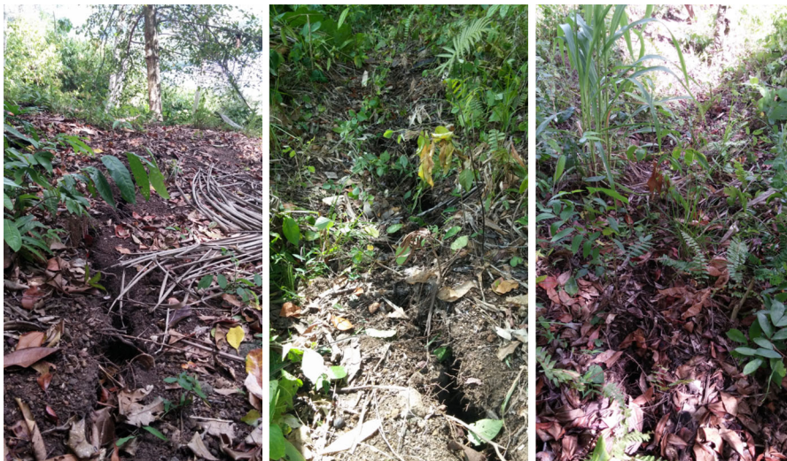
Fig. 9 Crack on the southern side of the mountain that might be indicative of future landslides
