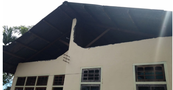
Fig. 6 Crack in residential buildings induced by the 2015 WHS
