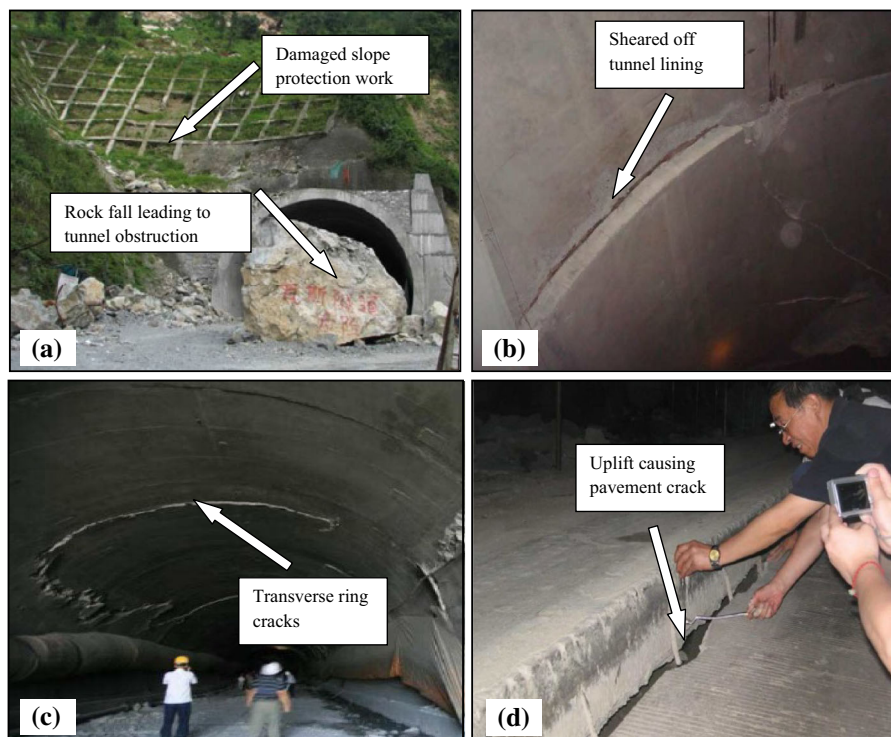
Fig. 5 Damages at Longxi tunnel during 2008 Wenchuan earthquake (modified after Tao et al. 2011): a Rockfall causing obstruction at tunnel entrance, b sheared off tunnel lining, c transverse ring cracks, d pavement cracks due to uplift
