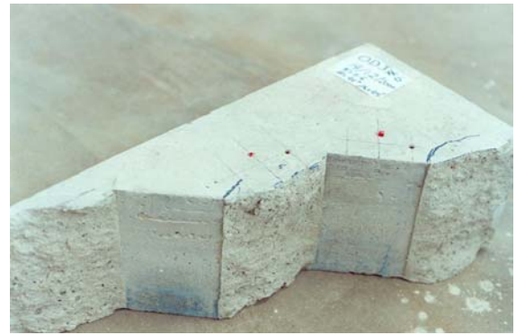
Fig. 2 Upper side of failure surface of specimen with \beta = 45^\circ and \alpha = 45^\circ cracks. (Mughieda and Alzo'ubi 2004)
