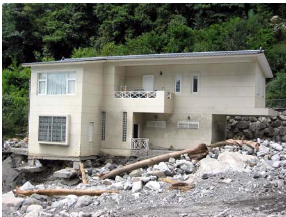
Fig. 4 Failure of foundation
