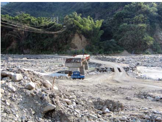
Fig. 21 Bridge lacked lateral resistance. Only three piers remained
