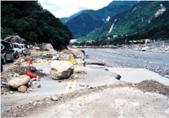
Fig. 12 Roadway failure due to scouring of road base
