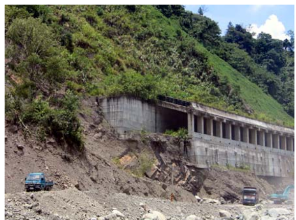
Fig. 24 Open tunnel destroyed by landslides
