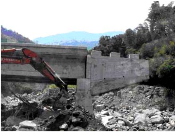
Fig. 25 An example of reinforced concrete abutment with-standing debris flow. Bridge approach has been washed away
