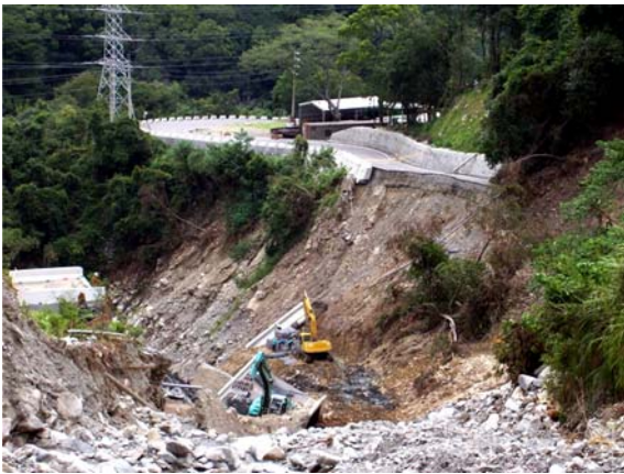
Fig. 13 Collapse of bridge and road
