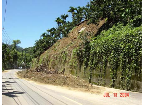
Fig. 7 Surficial slope failure
