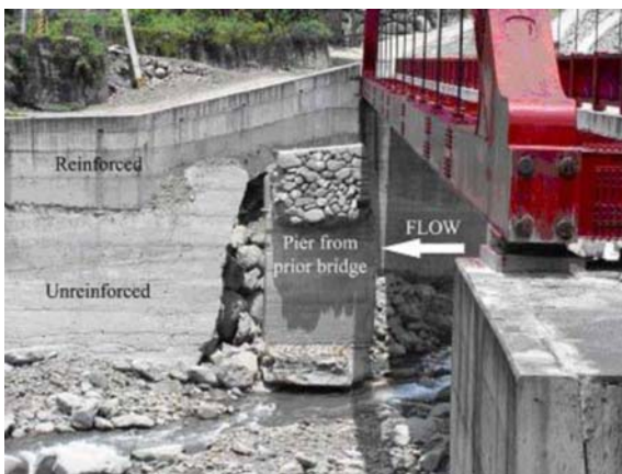
Fig. 26 Abandoned pier arrested debris on unreinforced concrete retaining wall
