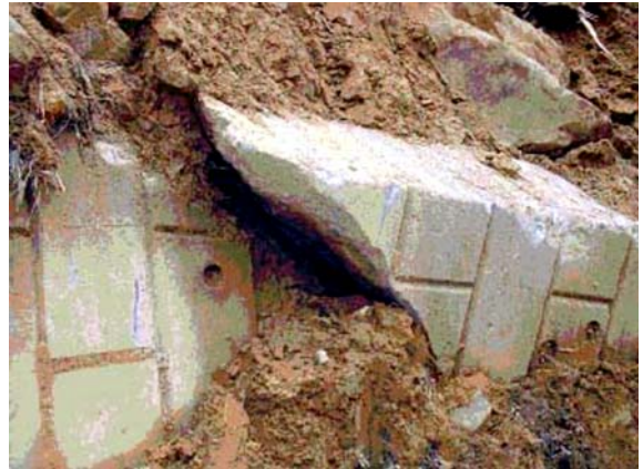
Fig. 23 Detail of failed unreinforced concrete retaining wall
