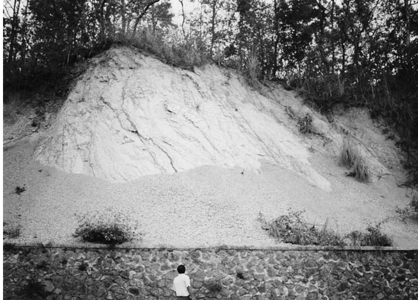
Figure 3. Rock falls in the roadside slope of Subang claystones resulting a thick mantle of regolith.
