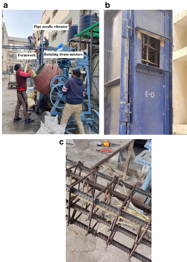
Figure 2. (a) The casting of RC columns. (b). Window opening in the formwork. ( c). Installation of thermocouples.
