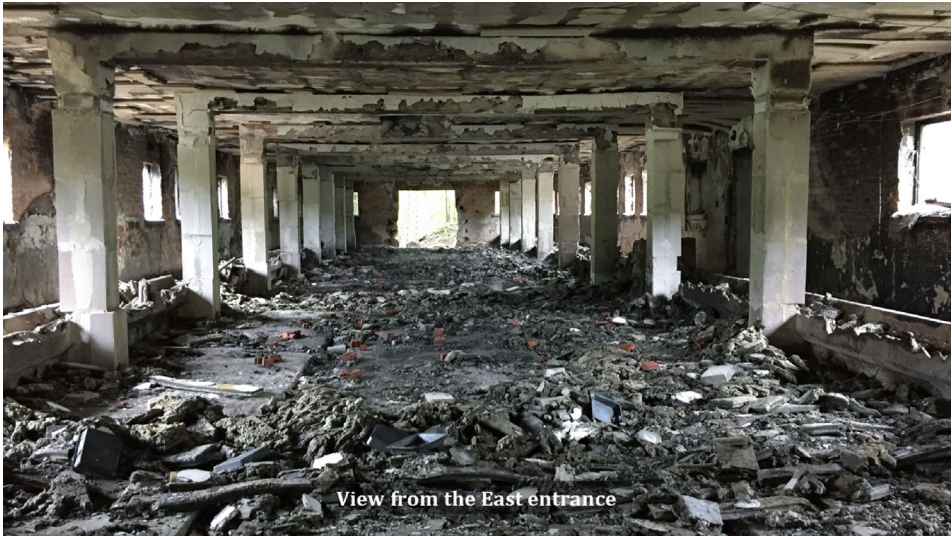
Figure 9. Illustration of the compartment after the experiment showing mineral wool protection which has fallen down from the ceiling and beams as fire progressed through the compartment.
