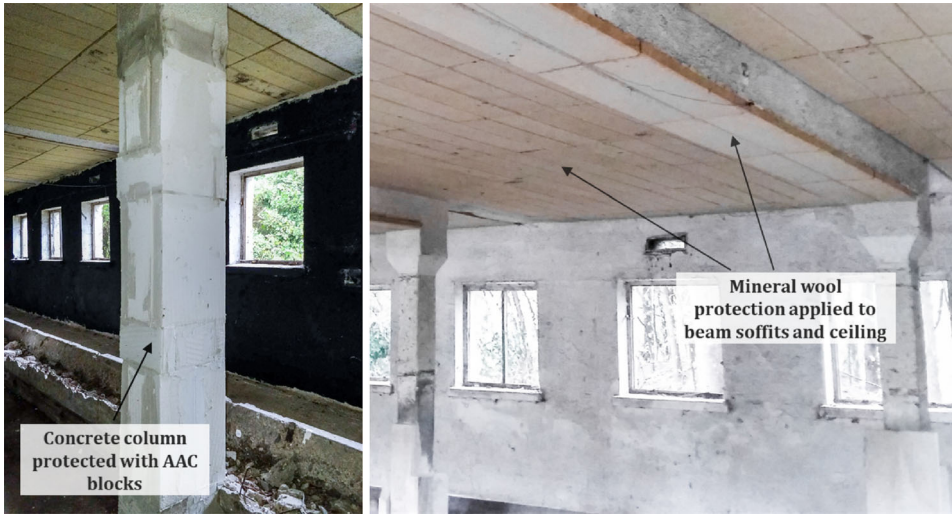
Figure 4. Final protection of the structure with autoclaved aerated concrete (AAC) blocks for the concrete columns (left), and mineral wool for the ceiling and beam soffits (right).
