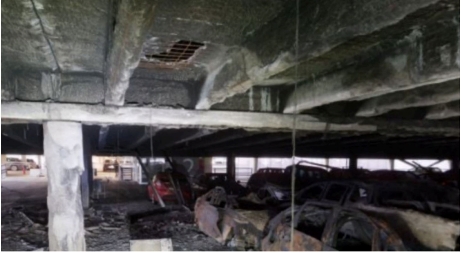
Figure 5. Concrete spalling in Stavanger, Norway 2020 fire [74].
