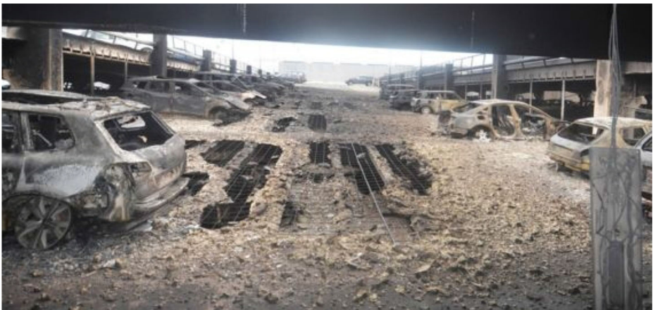
Figure 4. Concrete spalling in Liverpool, England 2017 fire [3].
