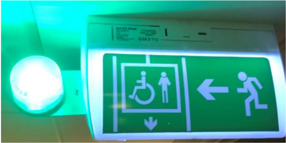
Figure 3. Flashing light attached to the evacuation sign pointing towards the elevator lobby.
