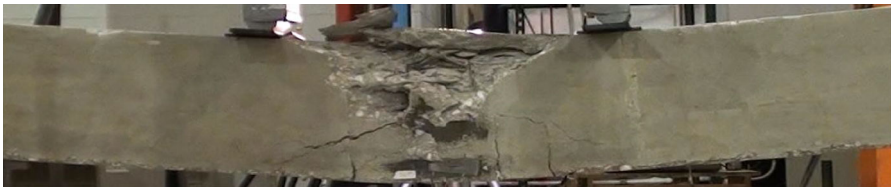
(c) Critical mid-span for beam B1 at failure
