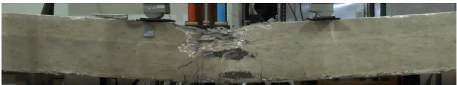
(d) Critical mid-span for beam B4 at failure
