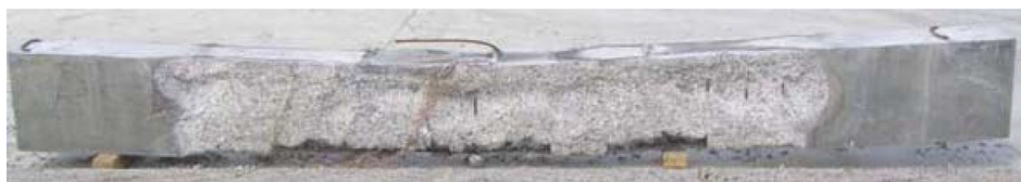
Figure 6. Spalling of HSC beam exposed to long fire [36].
