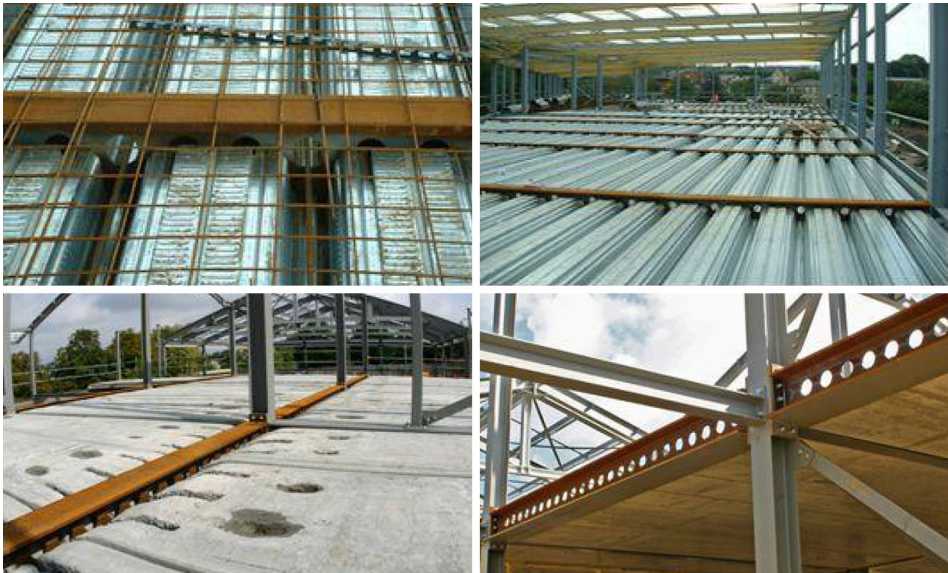
Figure 1. USFB used with profiled steel decking (top) and with pre-cast concrete unit (bottom) [13].
