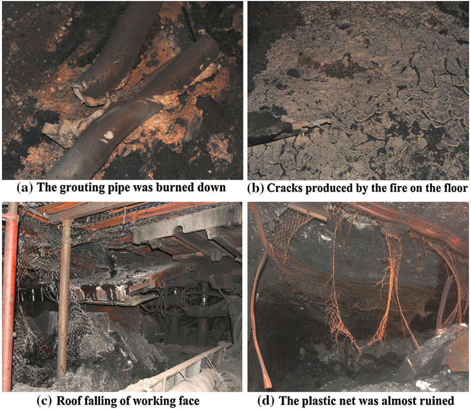
Figure 2. Fire results in the loss of the equipments surrounding the working face.
