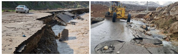
Fig. 3 Roads damaged by landslides due to intense rainfall ( https://www.irna.ir )
