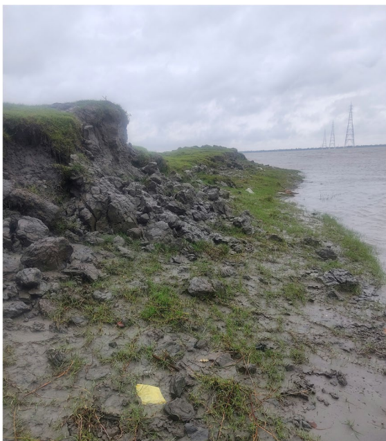
Fig. 23 Mud decoupling at the toe on the left bank near Akshyanagar
