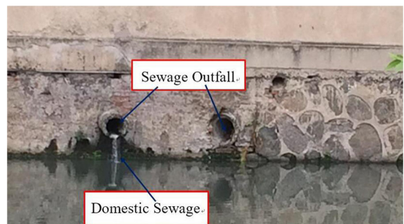
Fig. 10 Sewage outfall along the rivers
