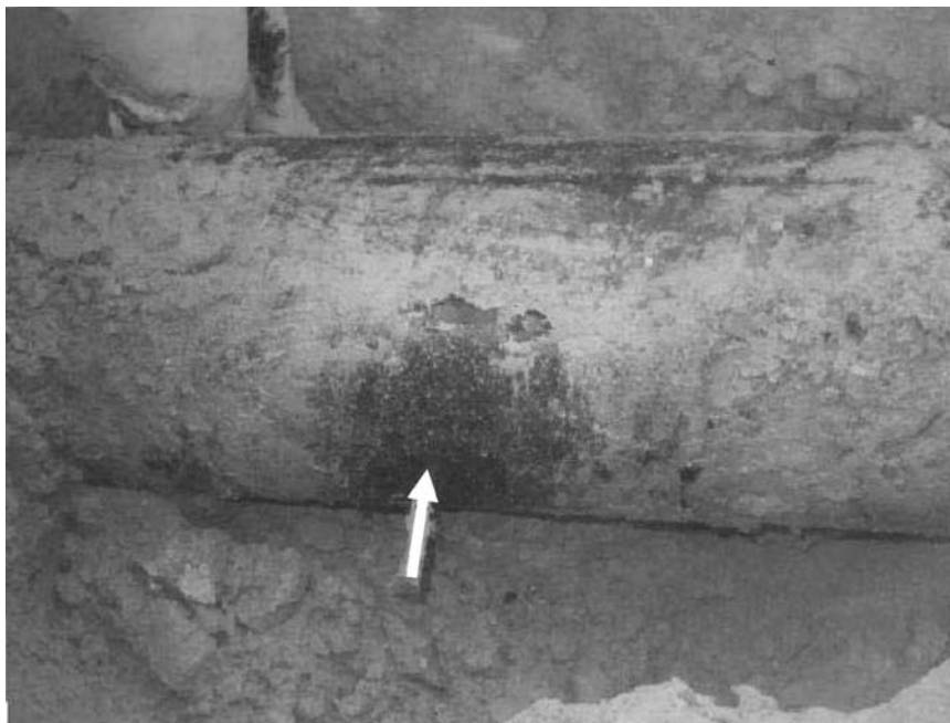
Plate 1. High pressure oil pipeline at Ogbodo-Isiokpo showing point of oil leakage.
