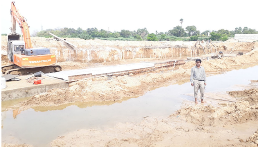
Fig. 12 Weir construction across the Thamirabarani River near Mukkani village by Tamil Nadu Public Works Department
