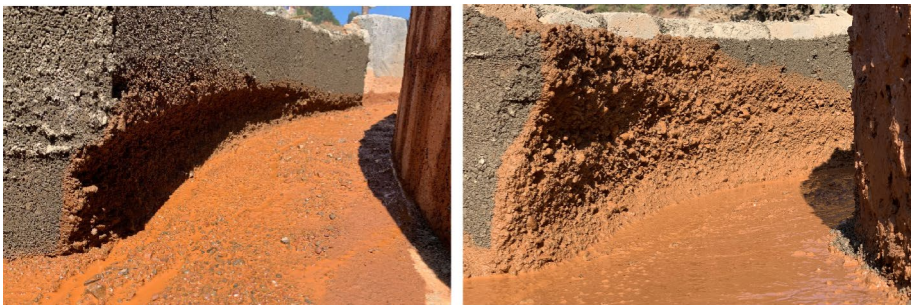
Fig. 5 Concave bank after erosion action, R_C = 2.7 m and 1.6 m respectively
