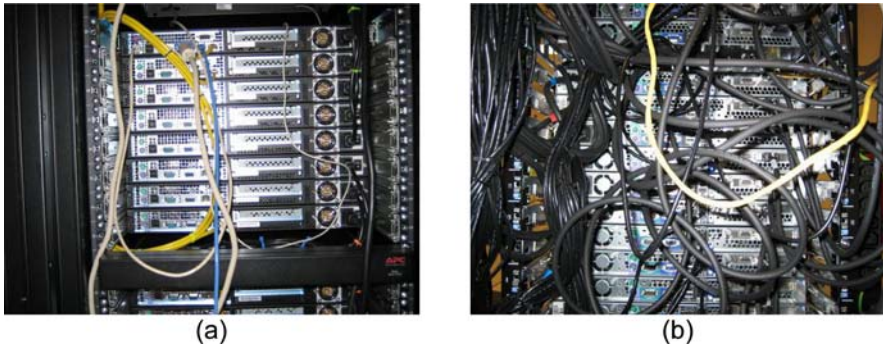
Fig. 7 Photographs of actual compute racks, showing (a) individual server fan and (b) rack cabling
