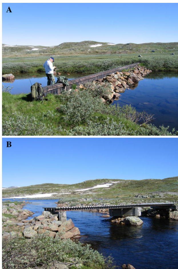
Fig. 2 The barrier (a) and the channel (b) constructed in 1952 to redirect a 12.4 km 2 drainage area away from the Veig river system to the Numedalslågen river system. For exact location of the constructed barrier and channel see Fig. 1. (Photos: Reidar Borgstrøm)
