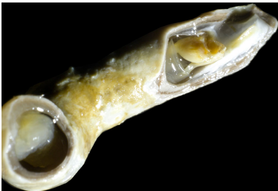
Fig. 5 Detail of the multi-layer tube of a frictioned Teredo bartschi . The sample was collected from the eroded intertidal portion of an Oak pile
