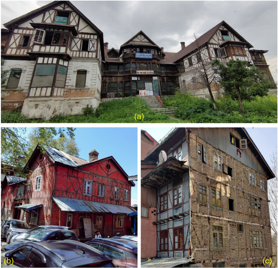
Fig. 1 Dhajji-Dewari structures in Kashmir, a a hospital building, b a government department building, and c a residential house
