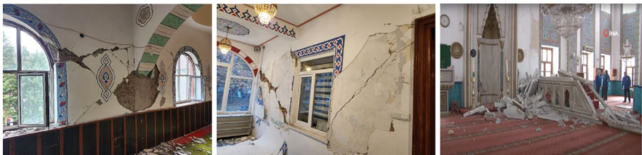
Fig. 10 Damage on the dome (left) and walls (middle) of Kiremitoğlu mosque, and damage to the interior of Düzce Cedidiye mosque (Anadolu Ajansı 2022)
