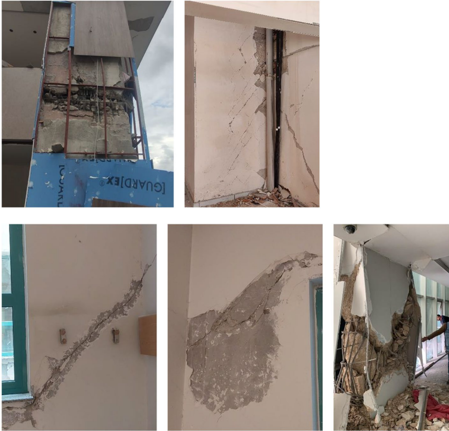
Fig. 12 Shear damage on columns
