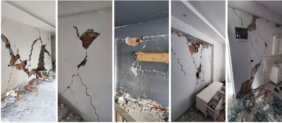
Fig. 16 In-plane infill wall damages
