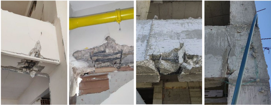
Fig. 8 Flexural damages on beams
