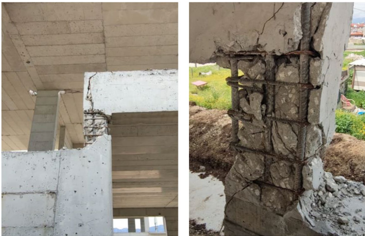
Fig. 11 Short column damage
