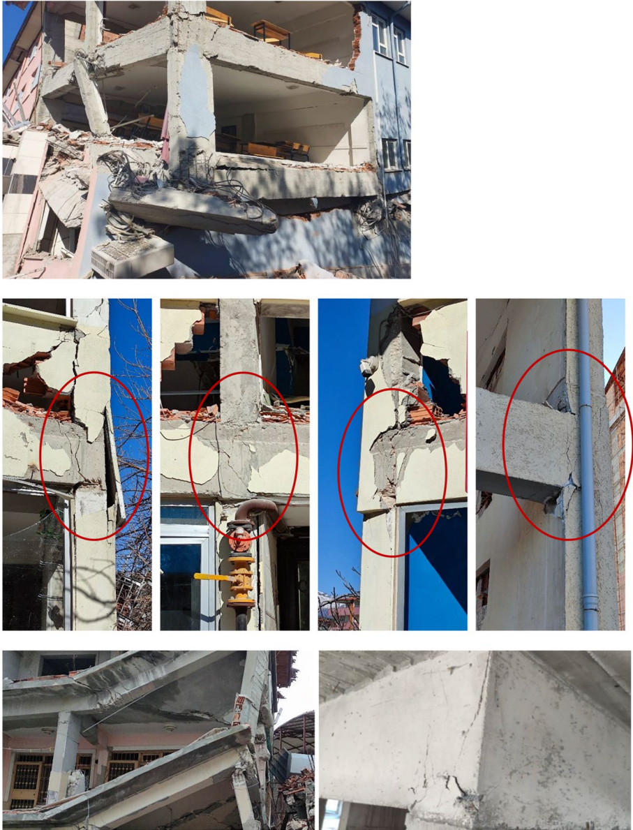
Fig.15 Shear damage on beam-column joint
