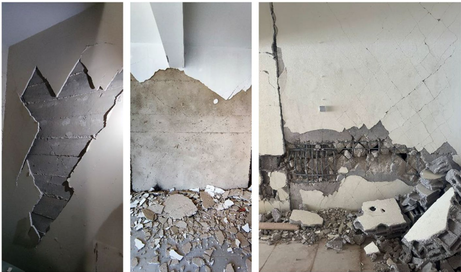
Fig. 14 Shear damage on RC walls
