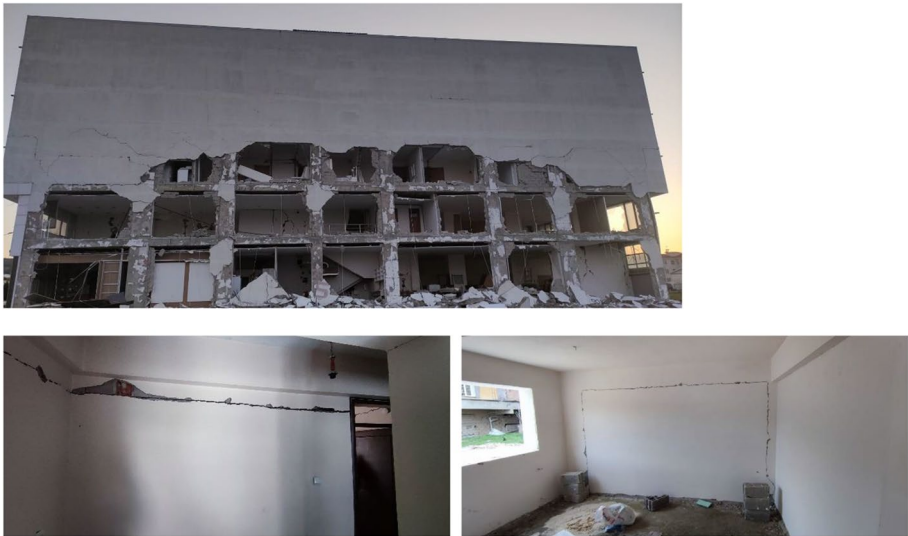
Fig. 17 Out-plane infill wall damages
