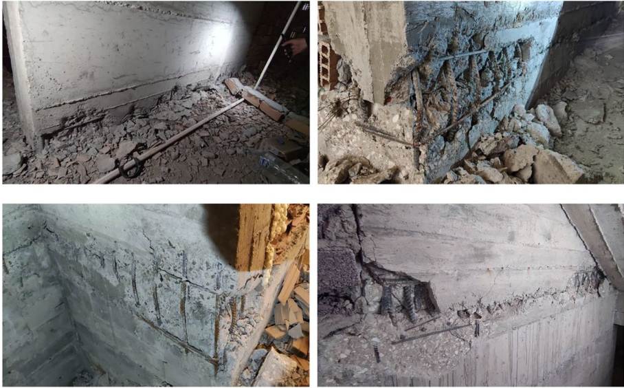
Fig. 13 Flexural damage on RC walls
