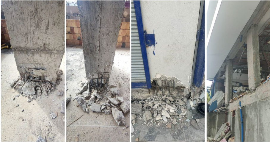
Fig. 10 Flexural damage on columns
