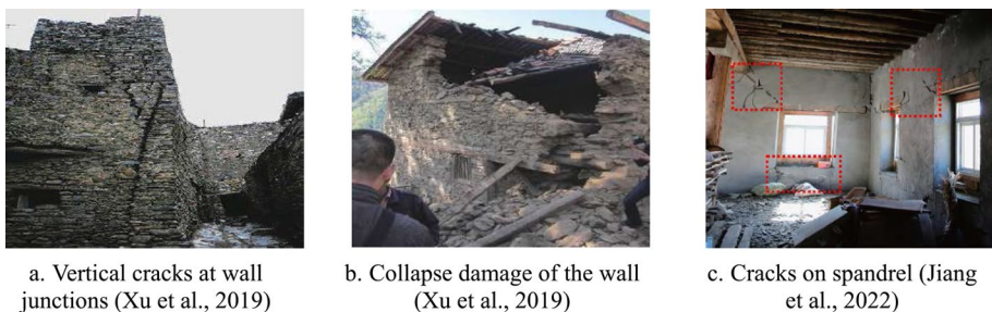
Fig. 2 Damage to Tibetan buildings (Jiang et al. 2022)
