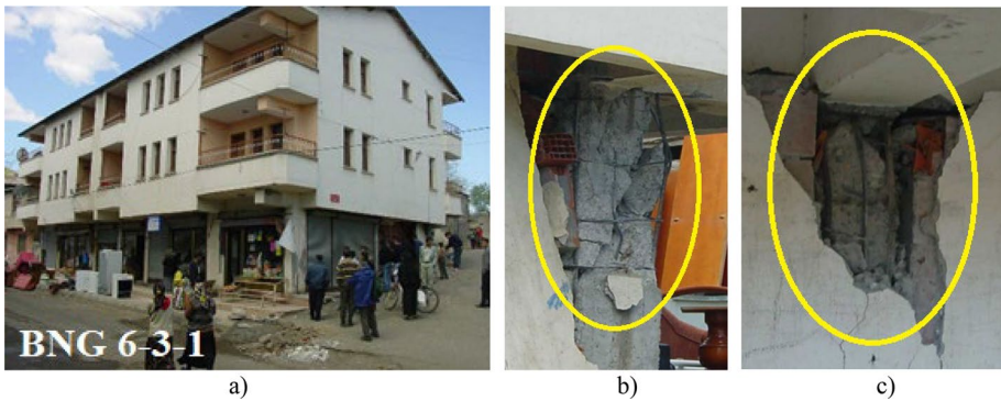
Fig. 22 a The BNG-6-3-1 building (heavily damaged), b Type D shear crack, reinforcement buckling, crushing of concrete core and rupture of transverse reinforcement, c Type D flexural damage with crushing of concrete core and buckling of longitudinal bars (METU 2003)
