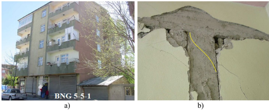
Fig. 19 a The BNG-5-5-1 building (lightly damaged), b Type A shear crack (METU 2003)
