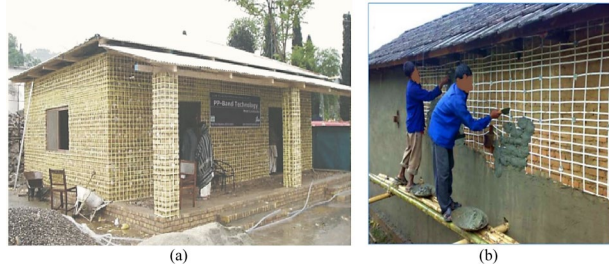
Fig. 4 Strengthening of the masonry building with PP band in Nepal (Macabuag et al. 2012; Heydariha et al. 2019)
