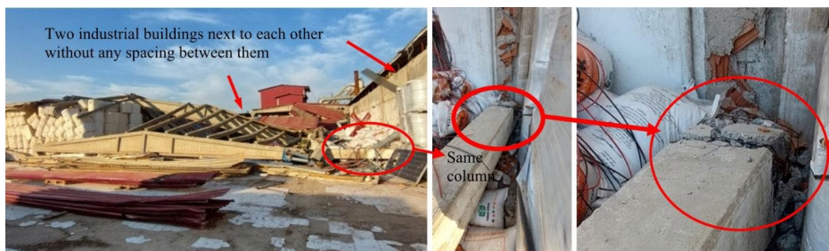
Fig. 8 Complete collapse of a precast RC industrial building in Turkoglu, as result of pounding effect
