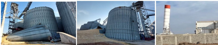
Fig. 13 Severely damaged or collapsed silos in Turkoglu, Kahramanmaras
