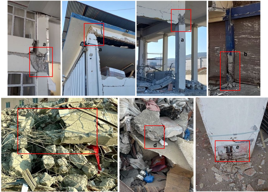
Fig. 11 Several failure reasons identified for the inspected RC facilities, such as (a) weak connections due to poor reinforcement detailing, (b) shear failures at the column ends due to large stirrup spacing (20–30 cm), (c) use of plain reinforcement, (d) use of improper aggregates in concrete structural elements, and (e) spalled concrete covers of columns due to severe corrosion
