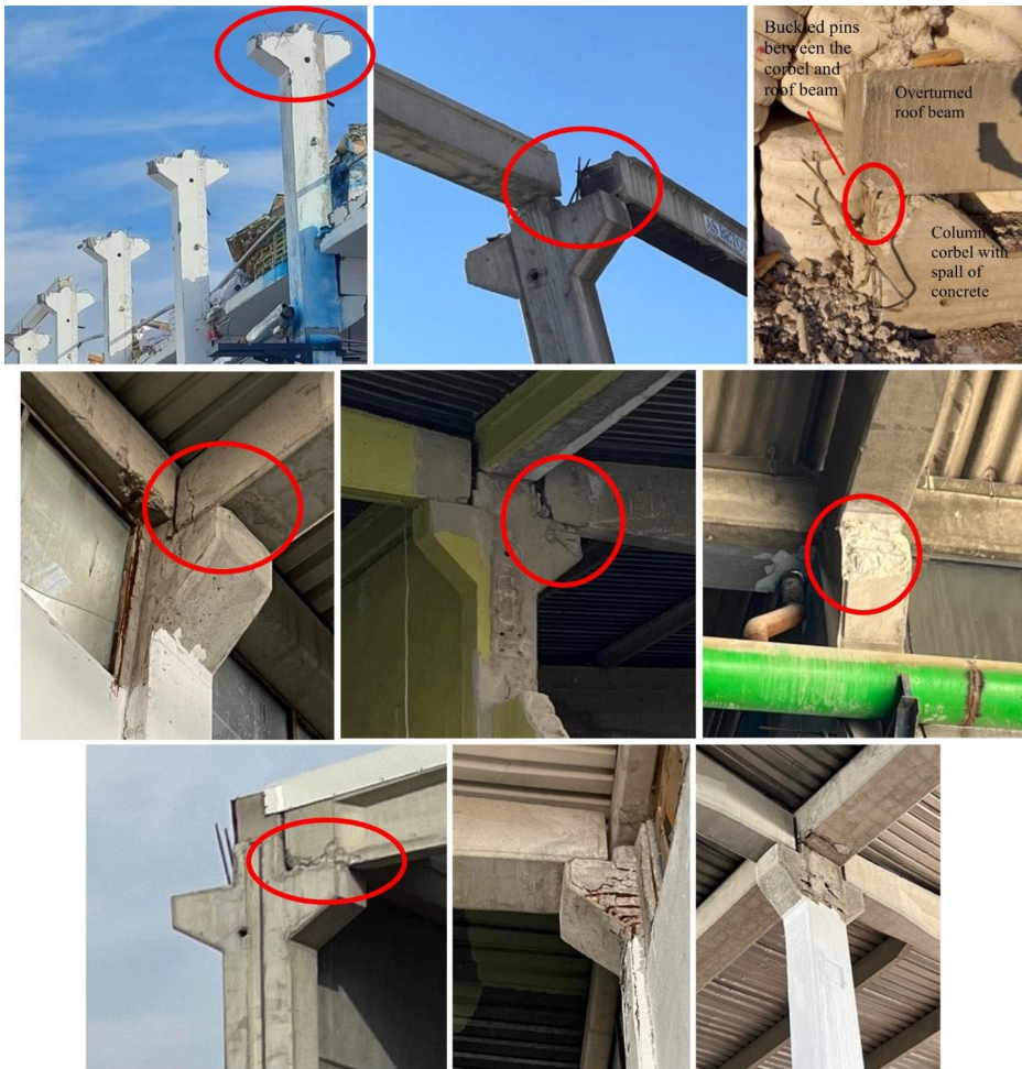
Fig. 7 Examples of pin failures on precast reinforced concrete industrial facilities located in Turkoglu (top); shear cracks and/or spalled concrete at corbels or roof beam ends observed in Adana, Nurdagi, Iskenderun, Turkoglu respectively (middle part from left to right and bottom-left); and severe corrosions observed on the elements (bottom-middle and right)
