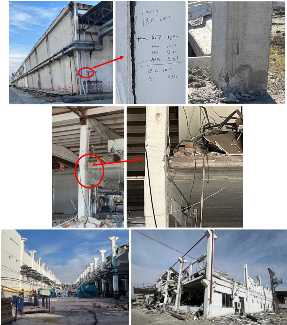
Fig. 6 Plastic hinges and flexural cracks observed at the column bases (top) and lateral support (middle); and complete collapses of roof systems together with main and supporting beams (bottom)
