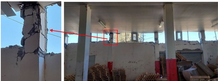
Fig. 12 Short column effects caused by the infill walls for a RC facility in Antakya (built in the 1970s)
