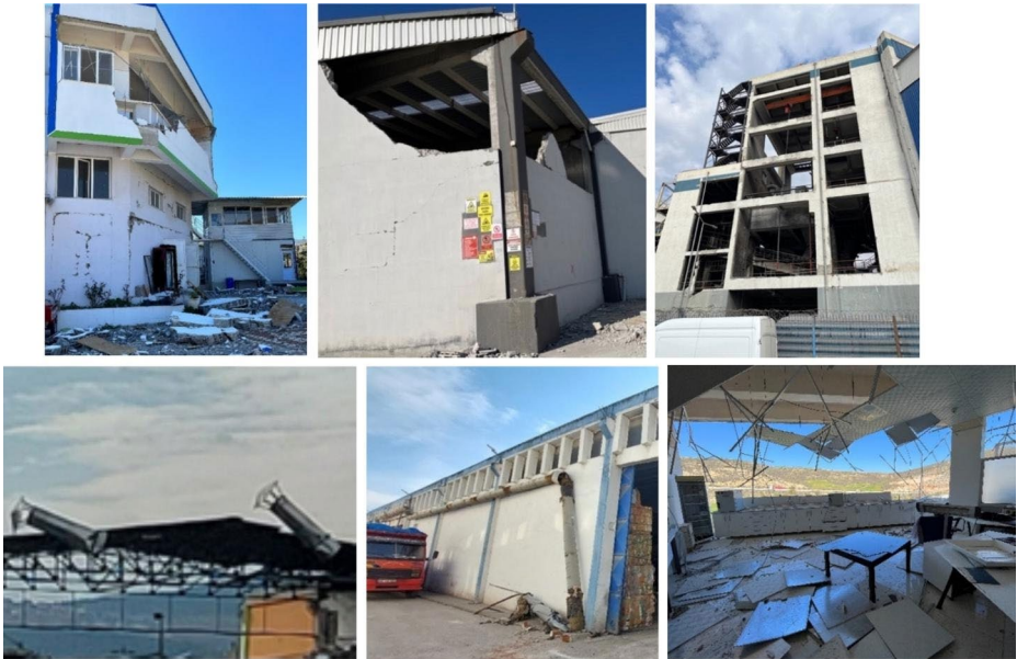
Fig. 14 Cladding/facade damages observed at the facilities in Antakya, Turkoglu, and Iskenderun (top, from left to right); and other observed nonstructural building damages such as overturned chimneys in Turkoglu, broken pipelines in Dulkadiroglu, and fallen ceiling panels in Antakya (bottom, from left to right)
