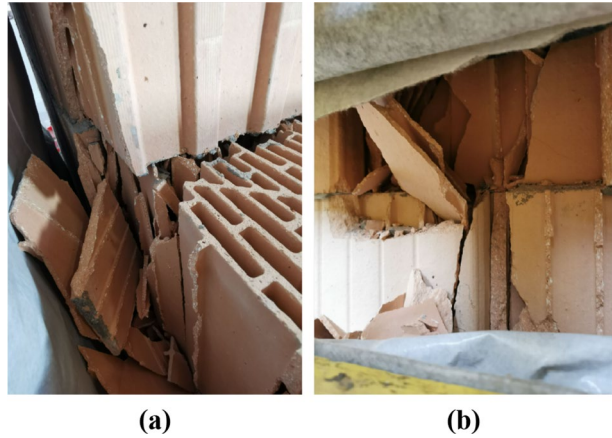
Fig. 6 Damage to the bricks from back side of the wall at 0.8% drift (a) and at 1.1% drift (b)
