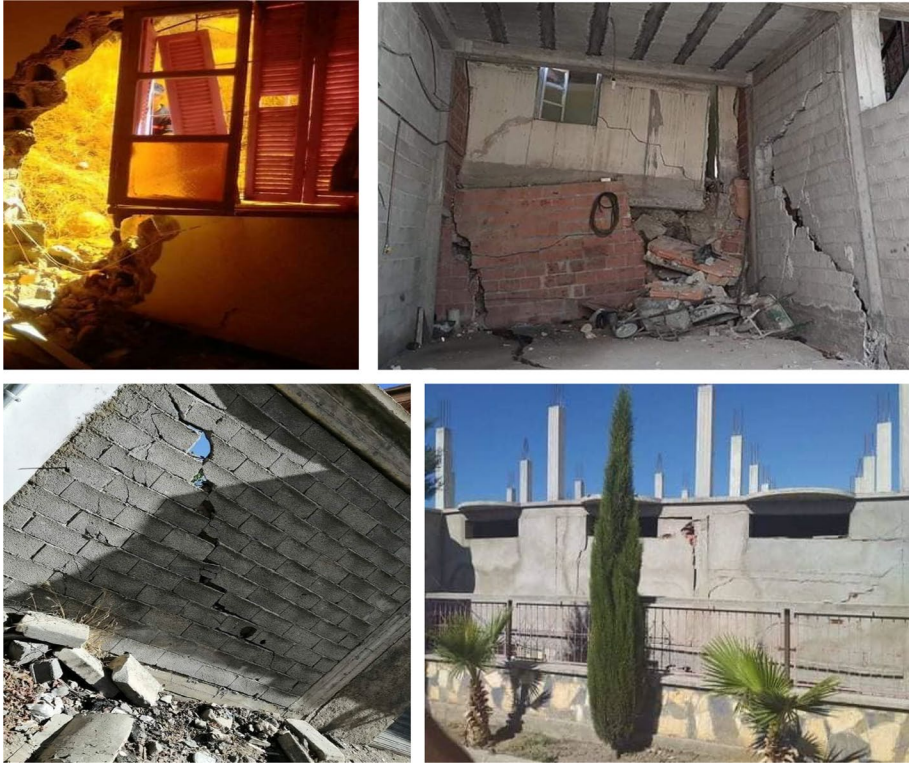
Fig. 16 Damage to partition walls
