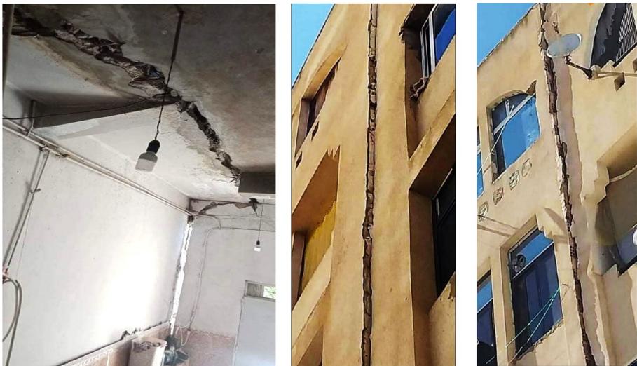
Fig. 19 Typical elevator shaft damage
