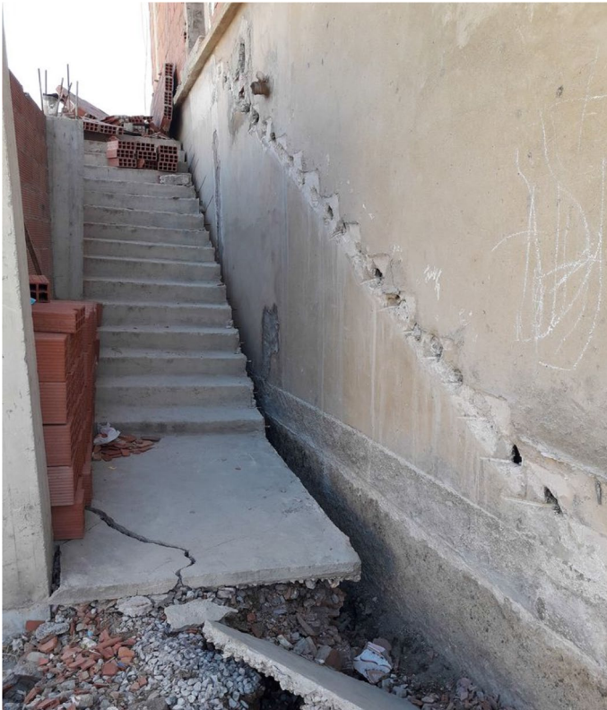
Fig. 18 Typical stairwell damage
