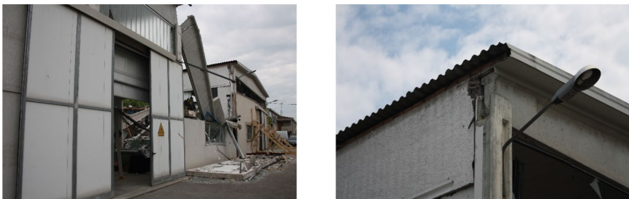
Fig. 12 Selected pictures of the post-earthquake situation (29/05/2012)
