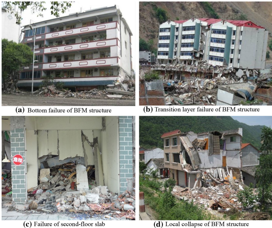
Fig. 6 Failure of BFM structure
