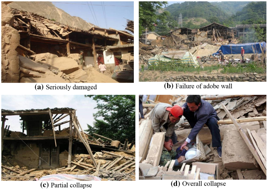
Fig. 2 Failure of adobe and timber structures
