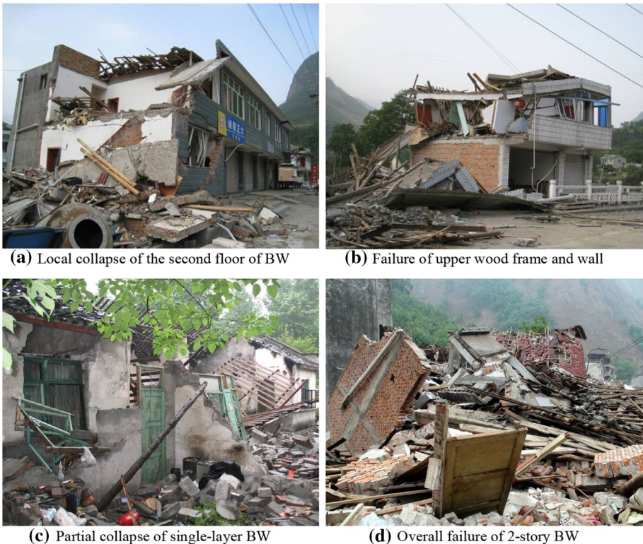
Fig. 3 Failure of BW structure (Li et al. 2021b)
