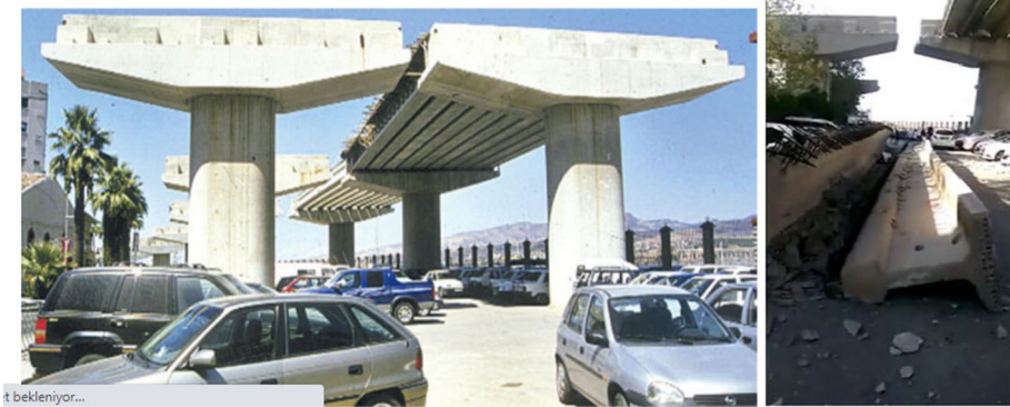
Fig. 22 An incomplete bridge construction 20 years ago without providing a lateral girder stability at the site (10 years ago and now)
