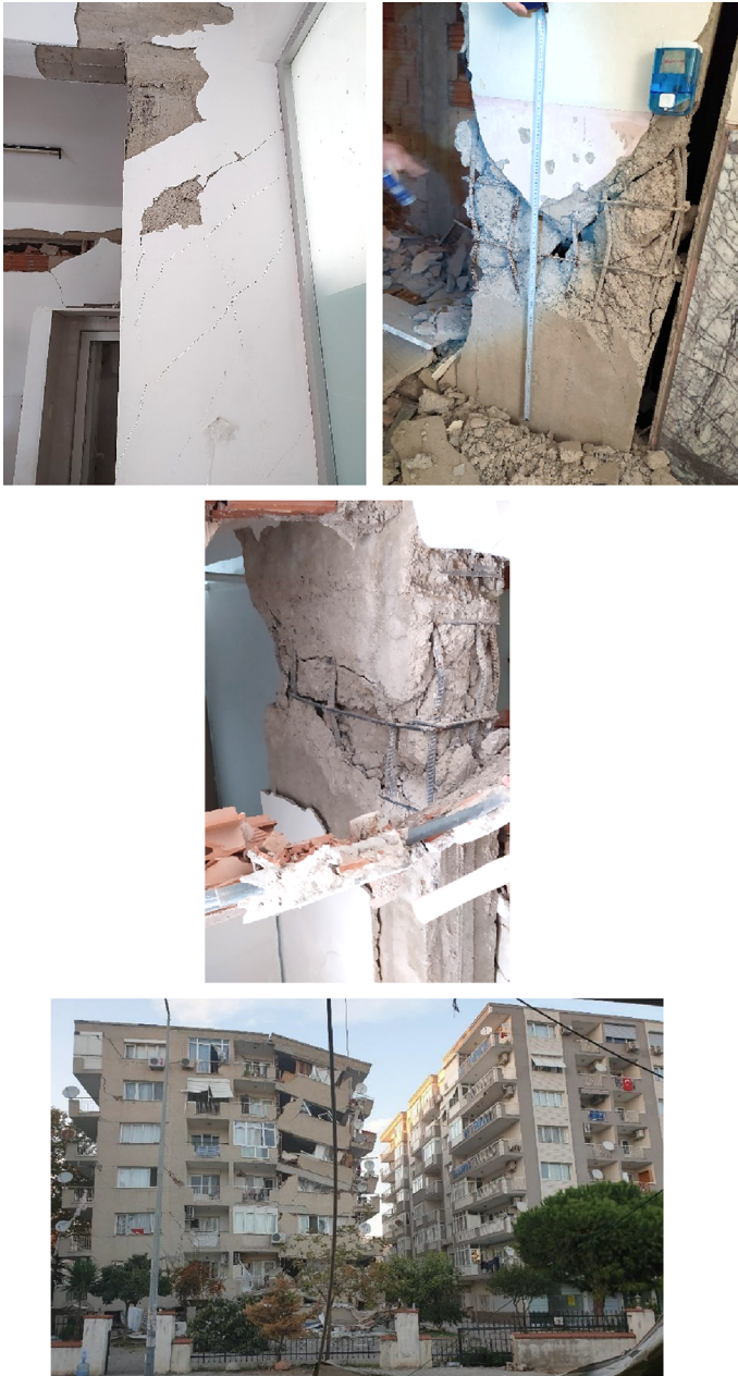
Fig. 11 Damage in the columns of two heavily damaged buildings
