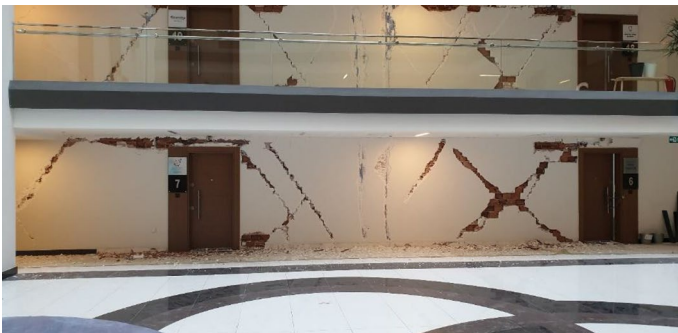
Fig. 13 Non-structural damage in infill walls due to large openings in the slab
