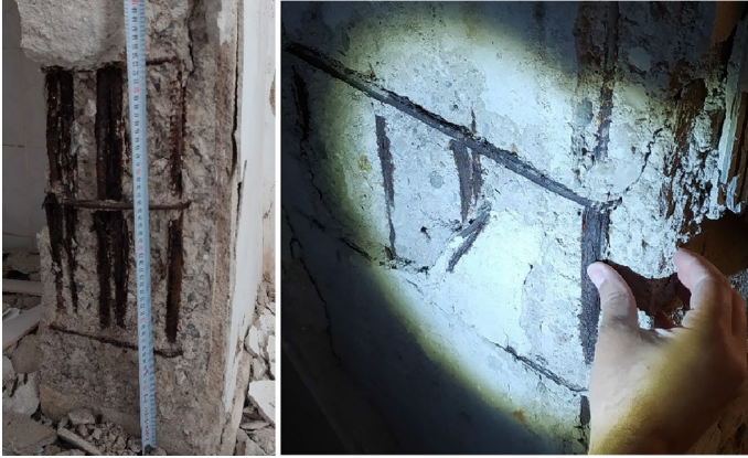
Fig. 12 Corrosion induced damages
