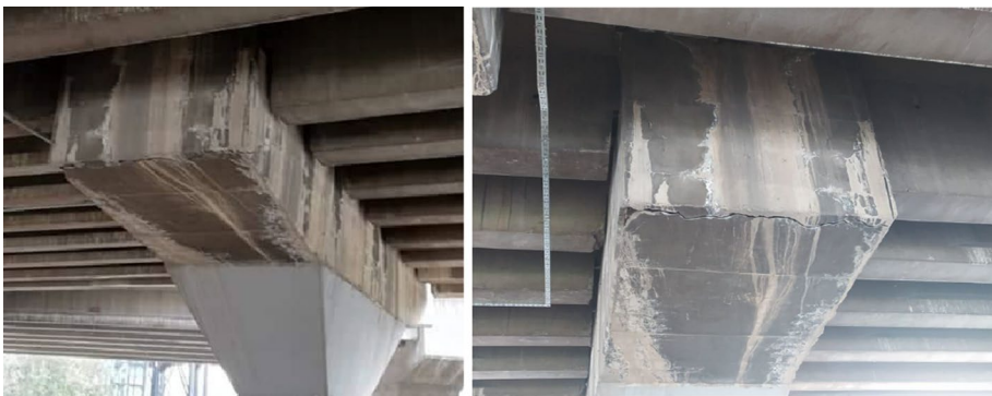
Fig. 19 A typical before-and-after earthquake photo (December 2019 and November 2020)
