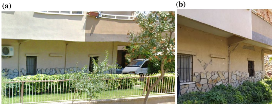
Fig. 9 Contribution of infill walls. a Before the earthquake (left), b after the earthquake (right)
