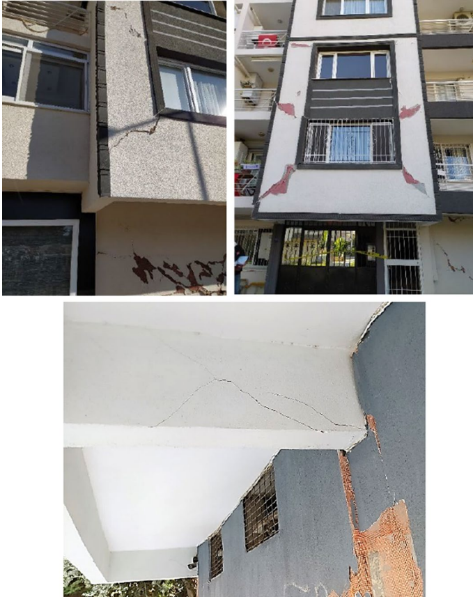
Fig. 10 Damage in overhangs
