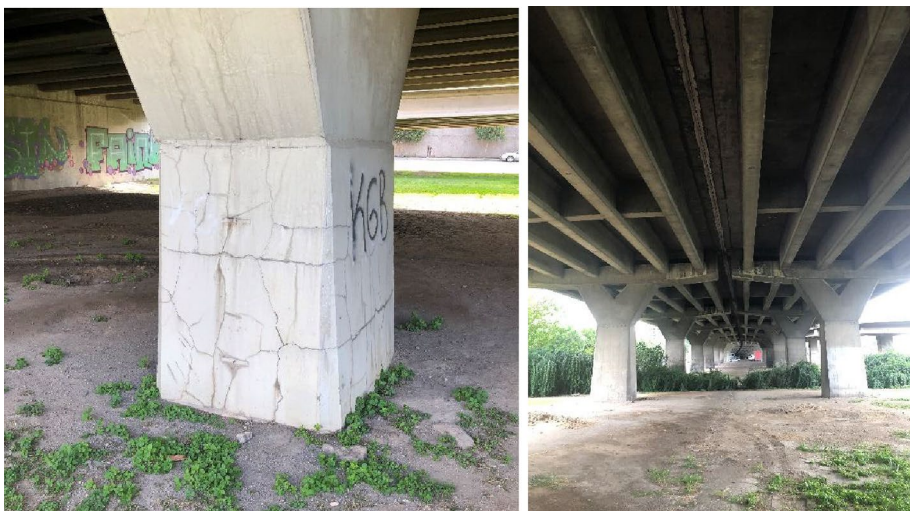
Fig. 21 ASR based cracks (non-seismic) and general view
