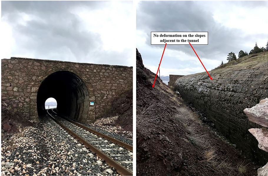
Fig. 39 A railway tunnel and rails exhibiting no damage ( 38^{\circ}28'52.8''\text{N} 39^{\circ}27'18.2''\text{E} /31.01.2020/15:08 & 38^{\circ}28'53.2''\text{N} 39^{\circ}27'18.4''\text{E} /31.01.2020/15:09)
