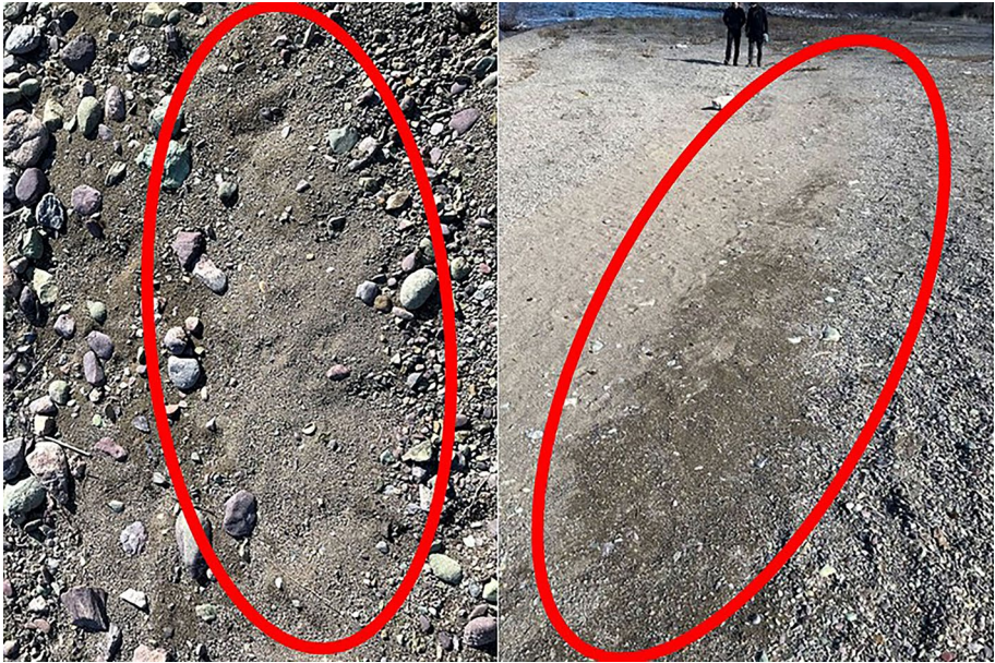
Fig. 12 Seismic soil liquefaction-induced sand boils at Kale shore ( 38^{\circ}25'15.2''N 38^{\circ}45'32.2''E/01.02.2020/12:32 & 38^{\circ}25'15.2''N 38^{\circ}45'23.9''E/01.02.2020/12:45 )
