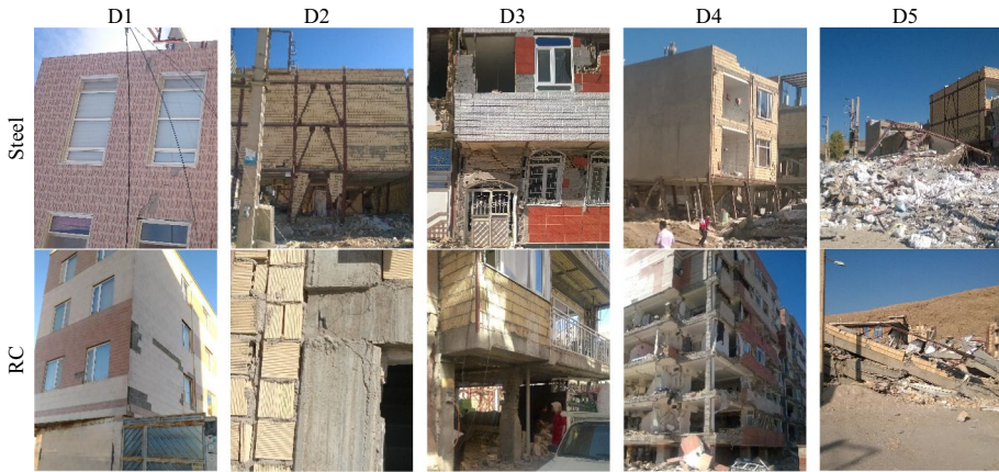
Fig. 1 Examples of damage grades to steel and RC structures during 2017 Sarpol-e-zahab earthquake
