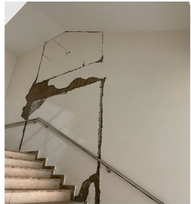
(b) Disconnection of wall from the frame (Sivrice township)
