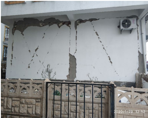
(a) In-plane damage (Ulukent district)
