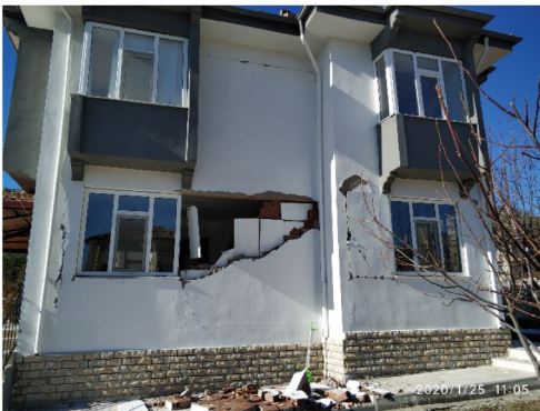
(c) Partial out-of-plane damage (Sivrice township)
