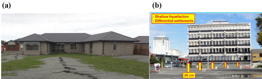
Fig. 10 a Type of damage on wooden; and b reinforced concrete buildings (from Cubrinovski et al. 2011c) (the yellow arrows in figure b represent the settlement distribution along the building)
