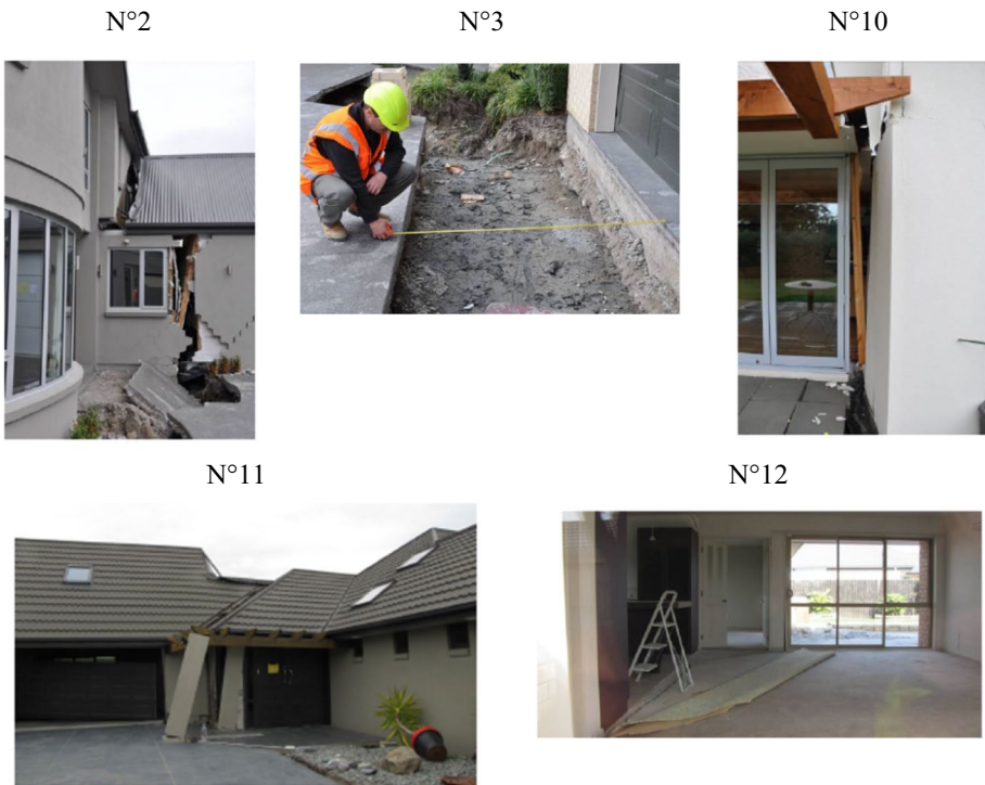
Fig. 20 Buildings B. Weak structures where the structural mechanism is developed
