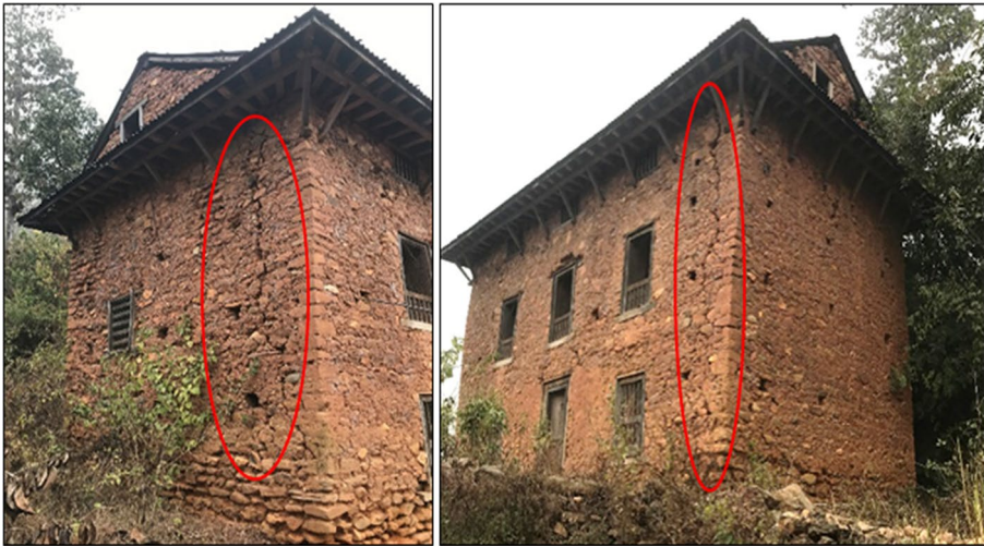
Fig. 19 Actual damage due to the 2015 earthquake in the case study PRE-SMM building from Sindhupalchowk district (vertical separation cracks have a maximum width of about 20 mm)
