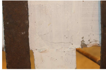
Story Drift = 1.10%: Occurrence of shear cracks in joint under connection closing.
