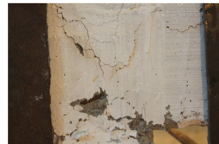
Story Drift = 3.73%: Concrete cover spalling at joint under connection closing.
