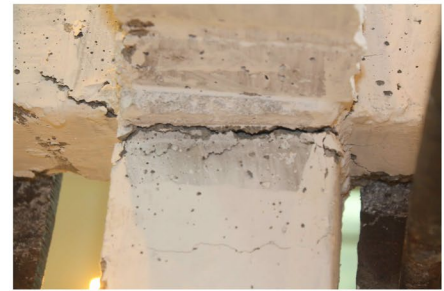
Story Drift = 2.50%: Extensive flexure cracking at the top ends of columns.
