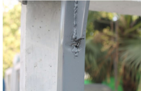
Story Drift = 2.82%: A small kink was seen in brace due to in-plane bending at brace end.
