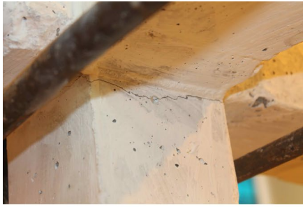
Story Drift = 0.30%: Flexure yielding at the top end of column under connection opening.
