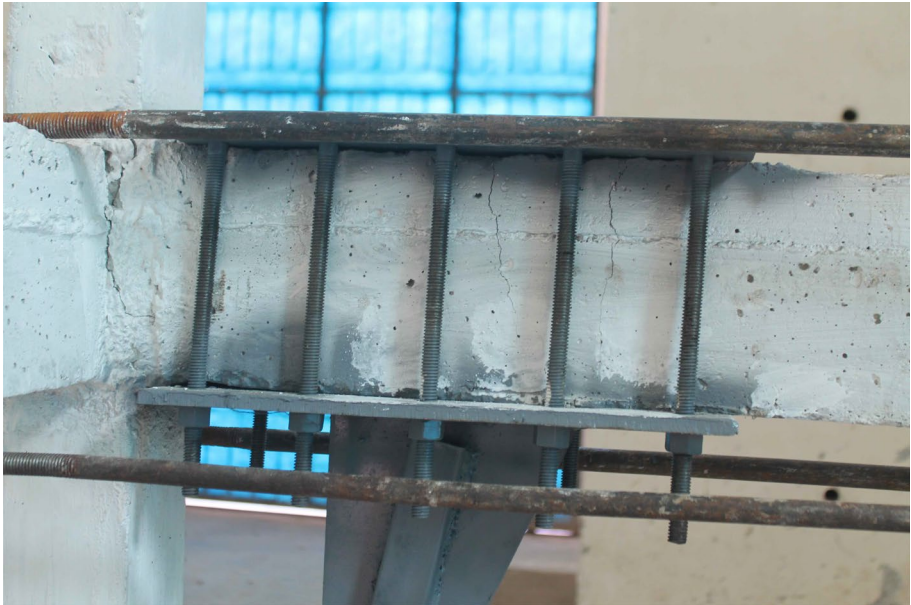
Story Drift = 1.94%: Distribution of flexure yielding over the beam length at the location of brace connection.
