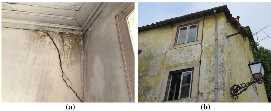
Fig. 4 Bad quality connections between orthogonal walls evidenced by diagonal cracks on internal walls (a) and by detachment cracks on the corners (b)
