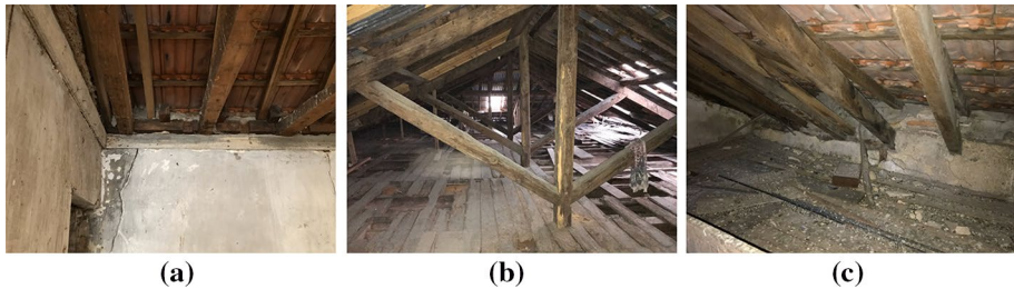
Fig. 5 Example of a two-order timber floor with connection to the perimeter wall (a), timber king post truss of a roof (b), mixed masonry-timber perimeter ribbon of the roof (c)
