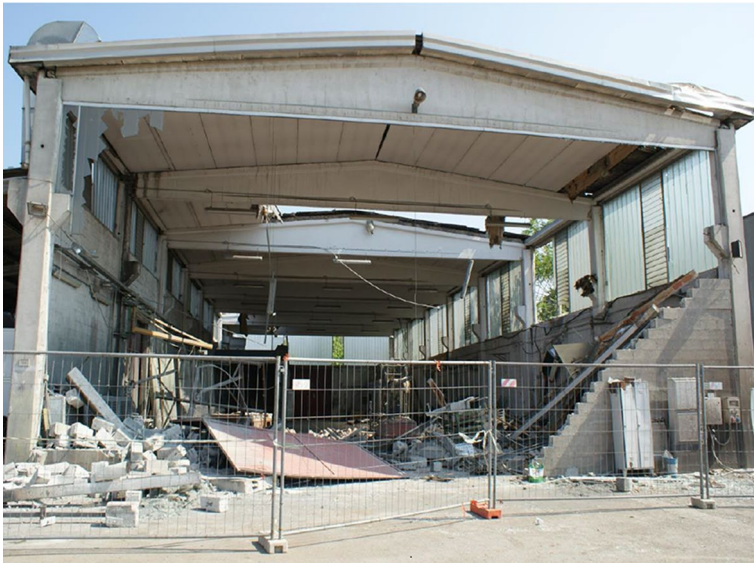
Fig. 1 Example of (precast) Long-Span-Beam building from SFINGE database, with widespread structural and non-structural damage. Source: Agenzia Regionale per la Ricostruzione—Sisma (2012)
