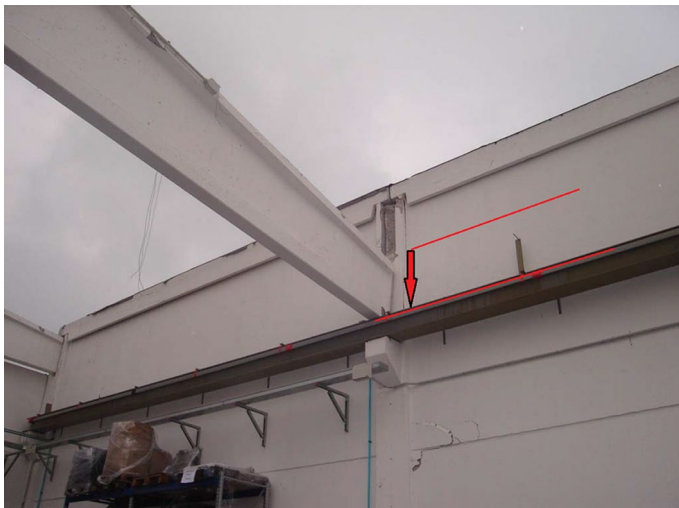
Fig. 4 Example of damage pattern P5—detail of a collapsed precast beam-column joint. Image source: Agenzia Regionale per la Ricostruzione—Sisma (2012)
