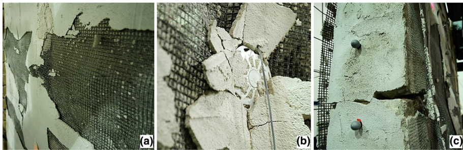
Fig. 15 Damage pattern of the reinforced stone wall at the end of the shake table test session: BTRM detachment (a), detail of the connector (b), local rupture of the basalt wires at the edges of crushed stones (c)
